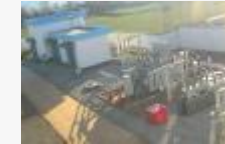
Power quality control device
